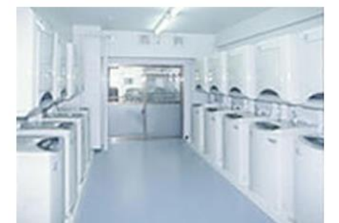
Laundry Room: Ten washer-dryer combos are installed.
